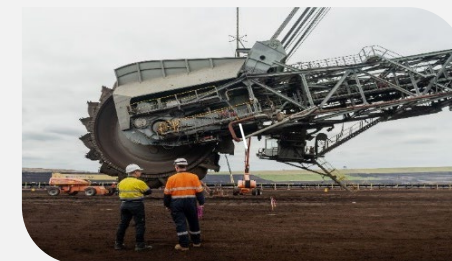
AGL Loy Yang Station Maintenance Industrial 5 Year Term
