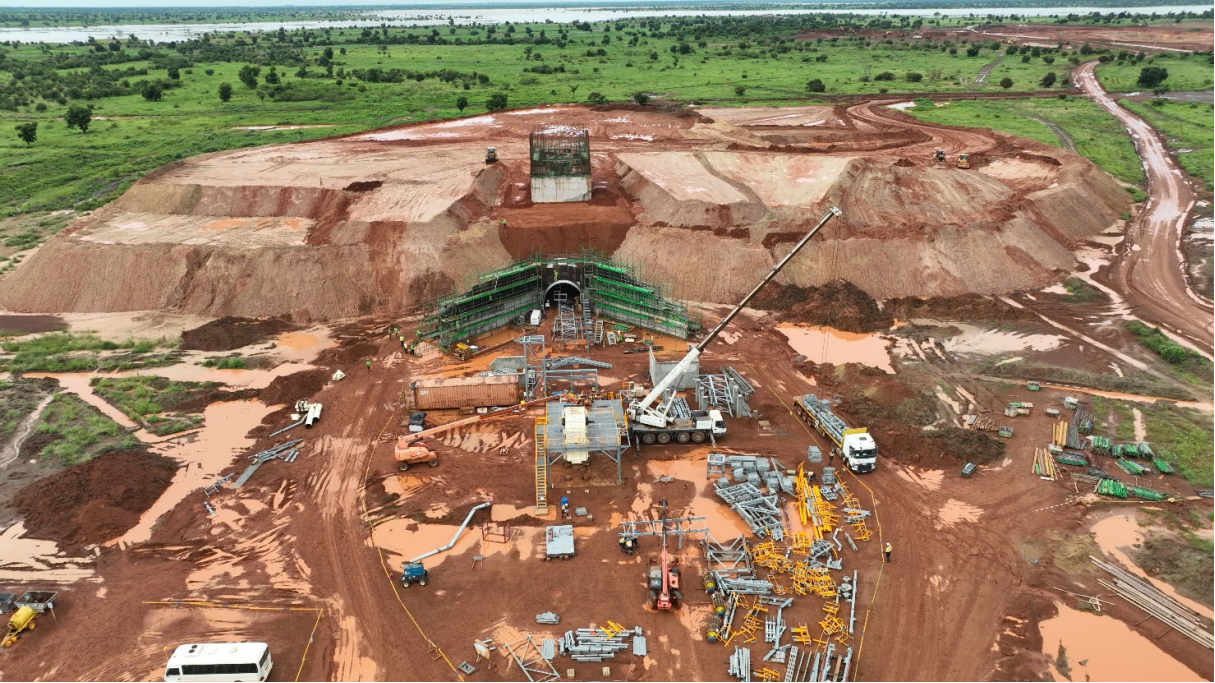
Kiaka Primary Crusher Area
