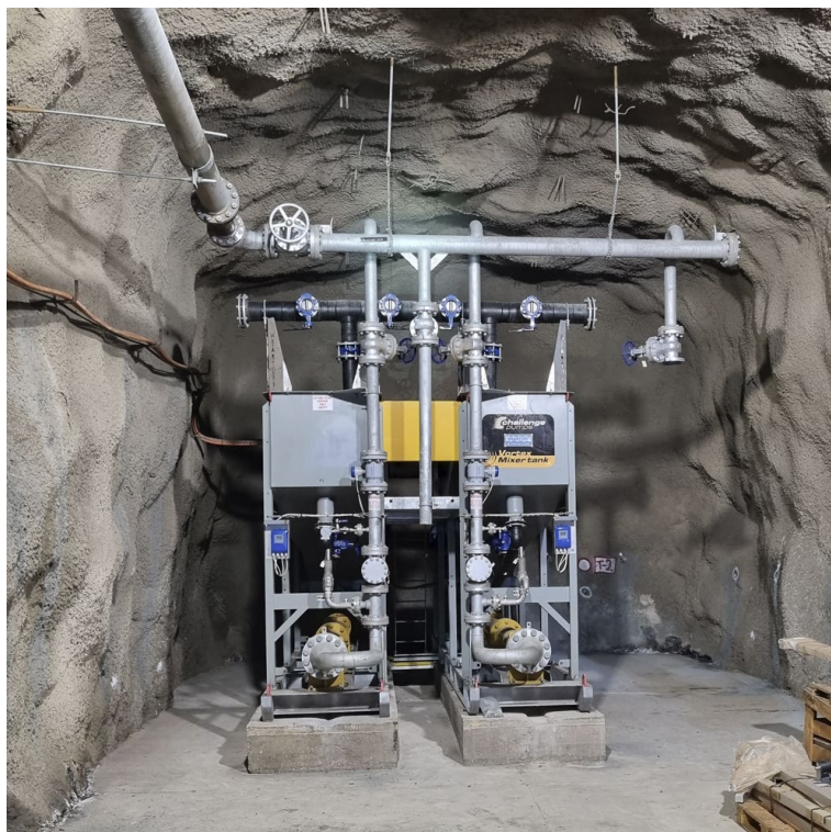
Figure 3: Recently installed and commissioned life of mine pumping station in the Viago 1230.
