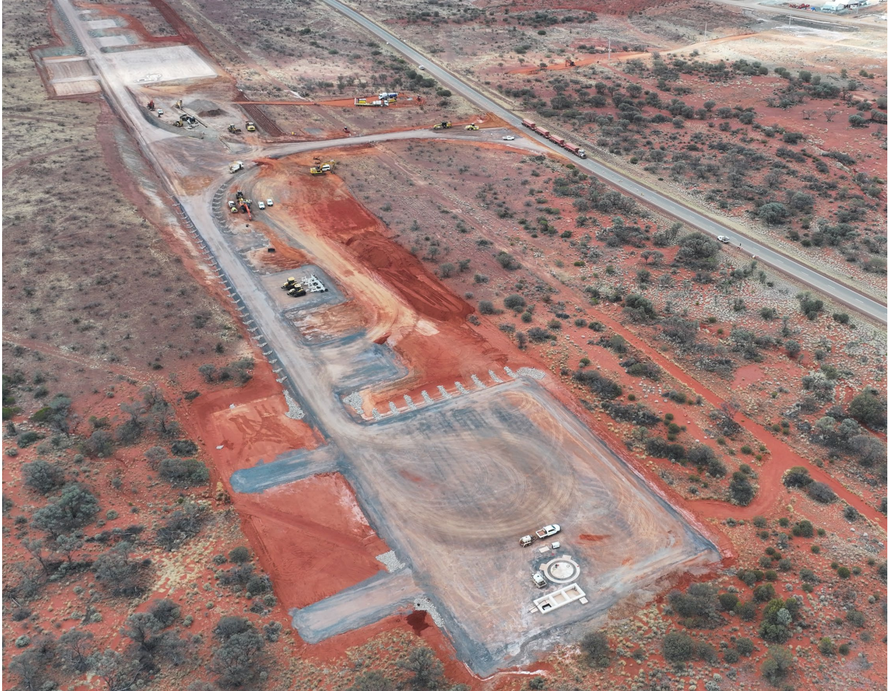
Figure 11: Earthworks and civils largely completed for the installation of 24 MW of wind turbines (4 x 6MW). Wind turbine components will be delivered to site commencing in November 2024.
