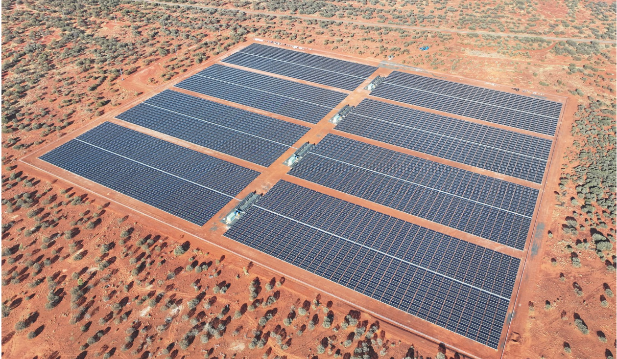
Figure 10: 27MW of renewable energy solar power complete and fully commissioned, providing ability to go “engine off” during the day.
