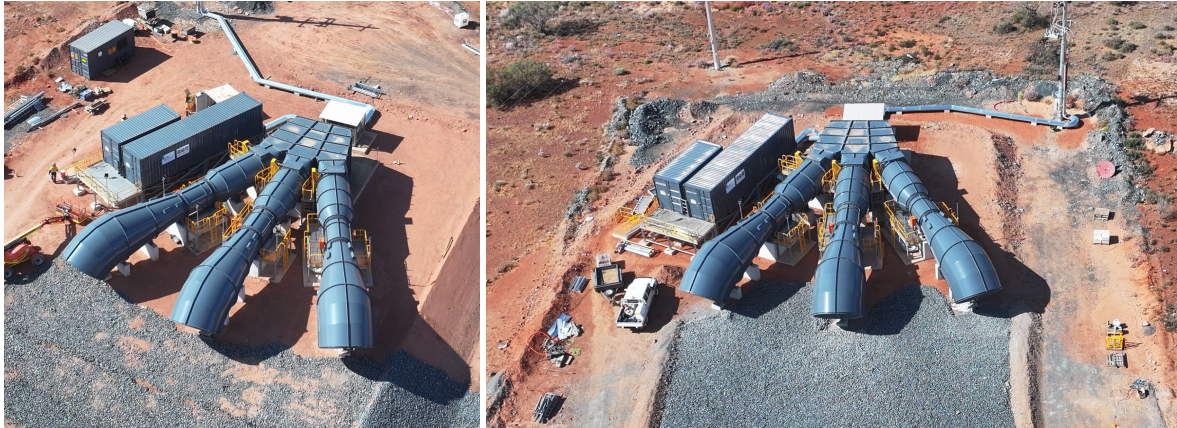
Figure 2: Two major ventilation installations commissioned in September 2024.
