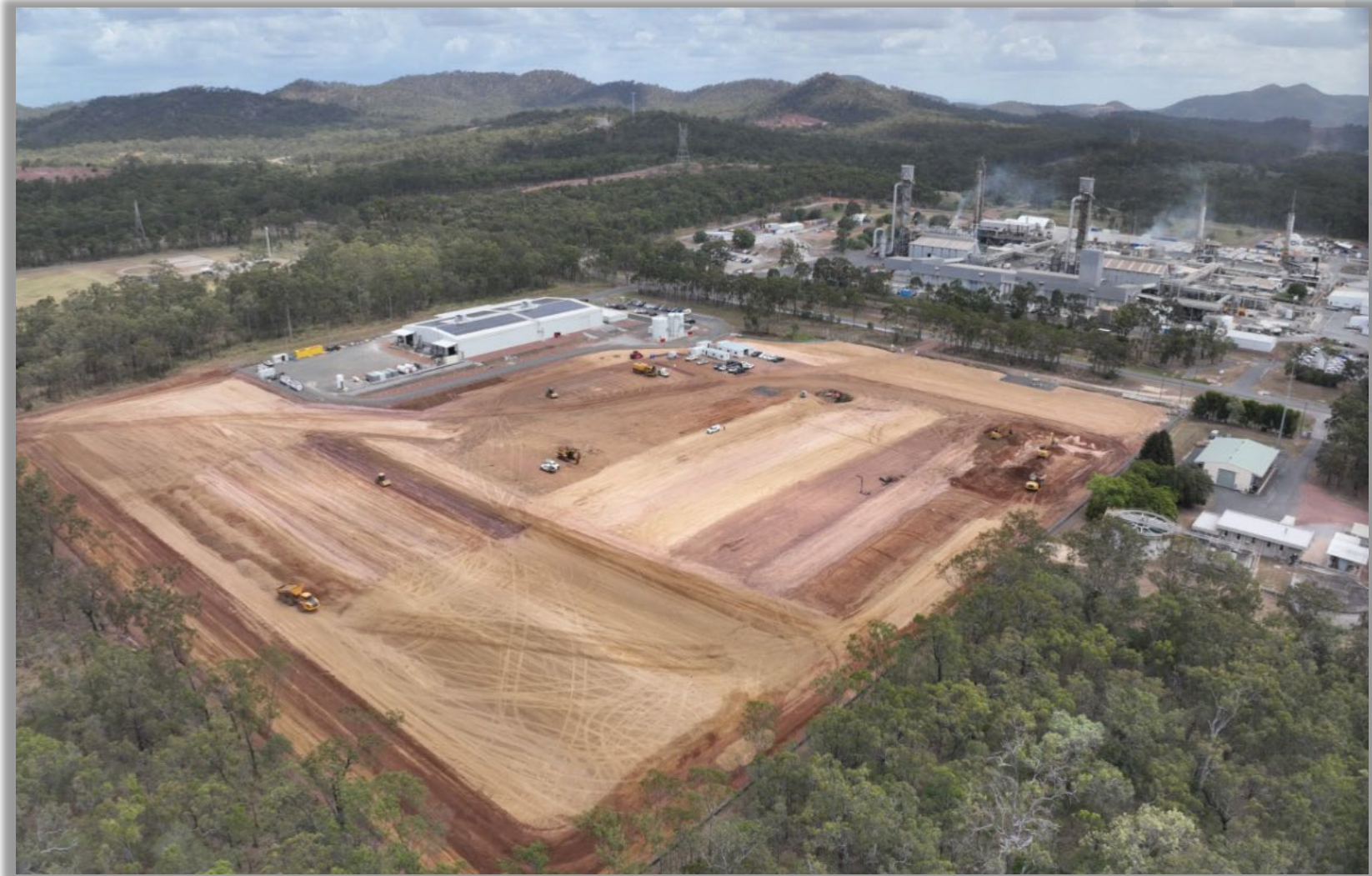
HPA First Project site looking southwest, showing earthworks well advanced, Stage 1 PPF and Orca Yarwun to the right of picture.
