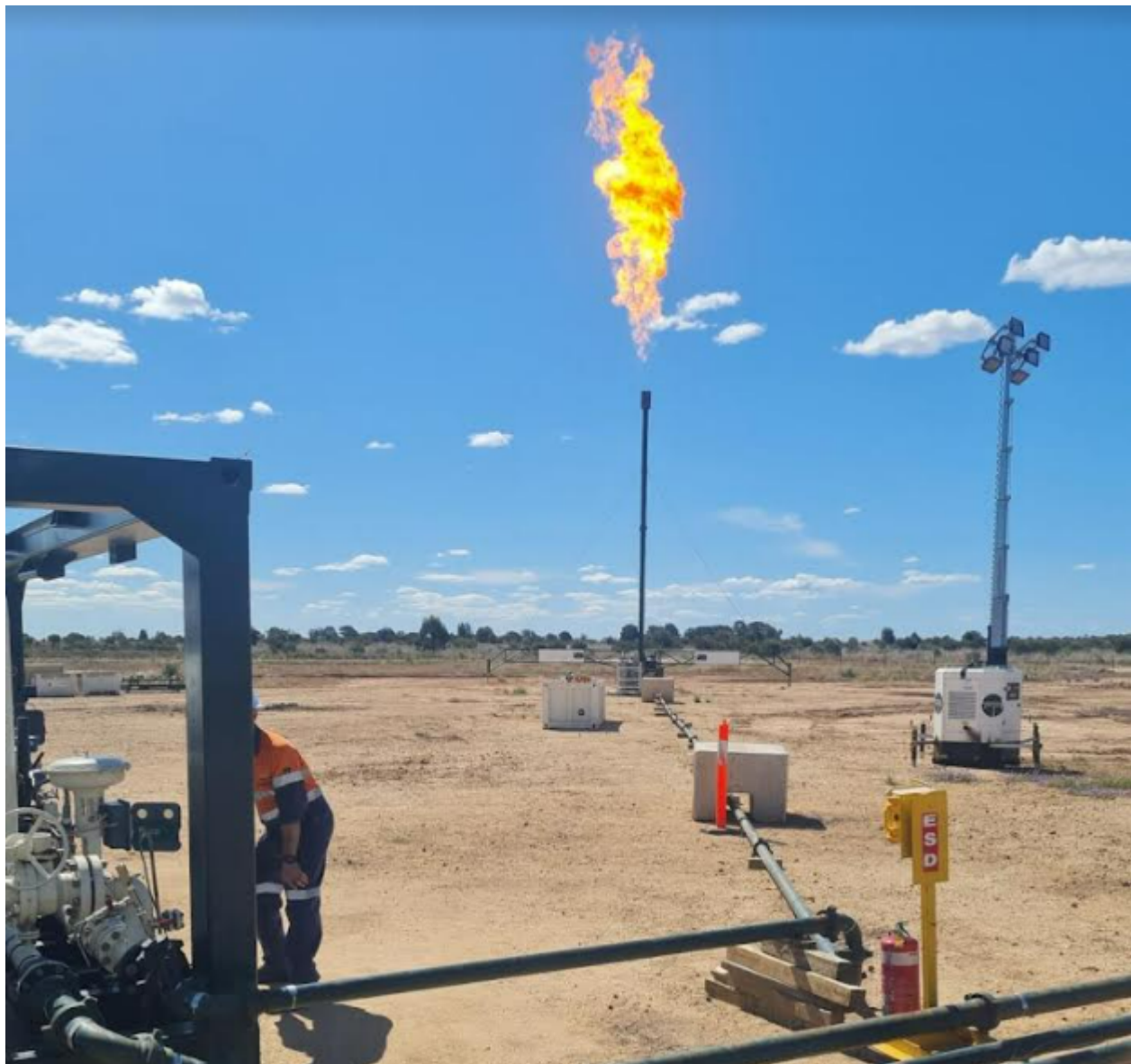
Flare from Daydream 2 prior to well being suspended
