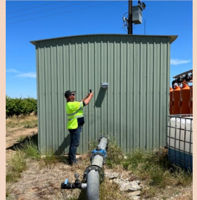
Entering a meter reading into the smart meter online portal to validate a smart meter installation.
