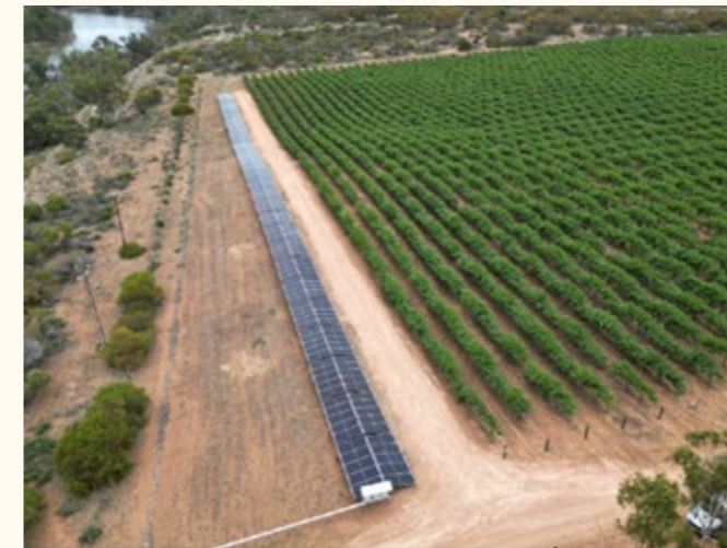
Solar panels installed at our Markaranka vineyard in South Australia.
