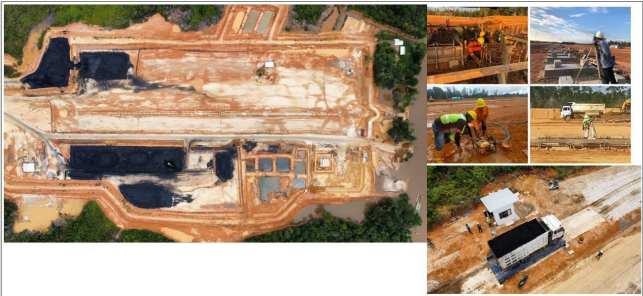
Jetty Batu Tuhup Development Progress (Weight bridge and foundation has been in place)
