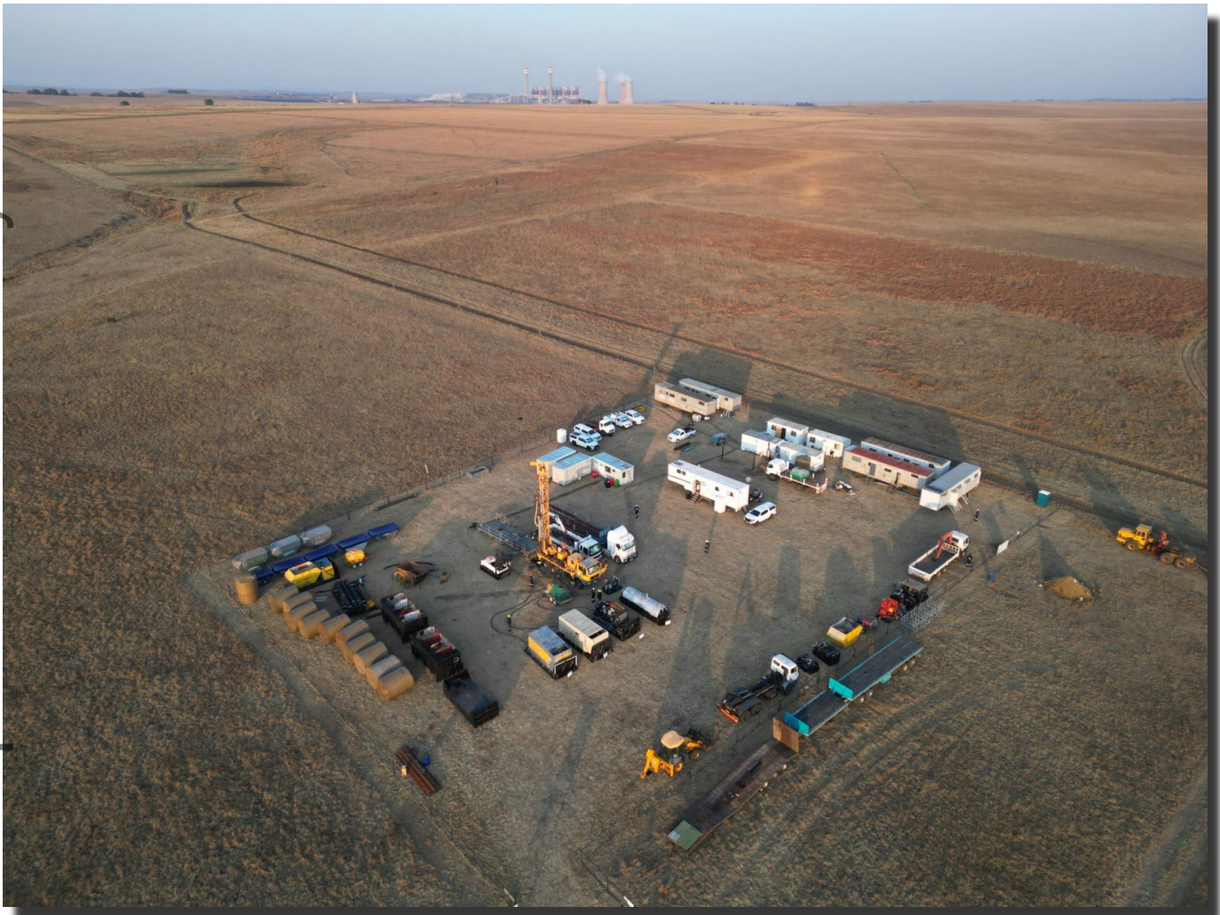
Figure 2 shows the production drilling rig on site for spudding well 271-23PT with Majuba power station in the background.
