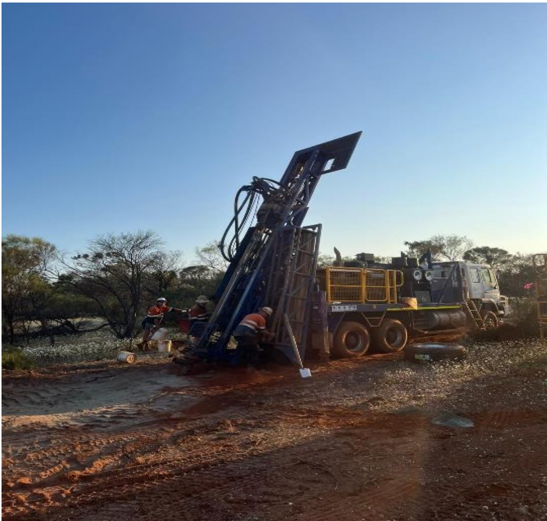
Picture 3: Ragland AC rig on site at Wildflower (First Hole this morning).
