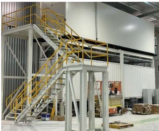
Classifiers MCC (upper level)
