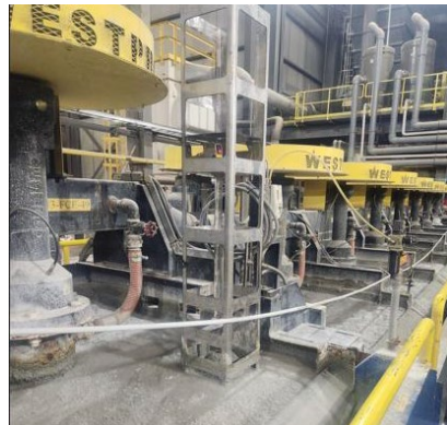
Picture 2: Mechanical slurry level measurement
