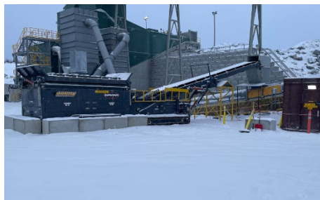
Picture 2: Temporary feeder system
