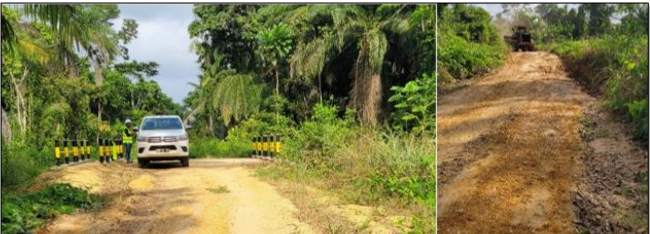
Figure 3 – Site access roads to the Cácata mine site being re-grated and upgraded.
