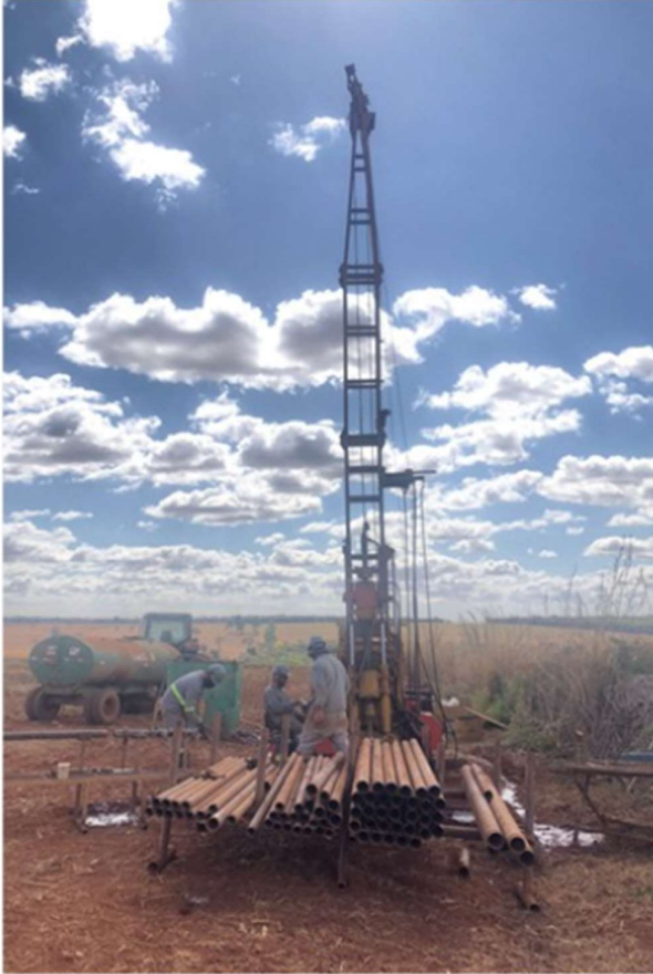
Figure 1: Diamond drill rig at DD 008 drill pad during operation in Coda North
