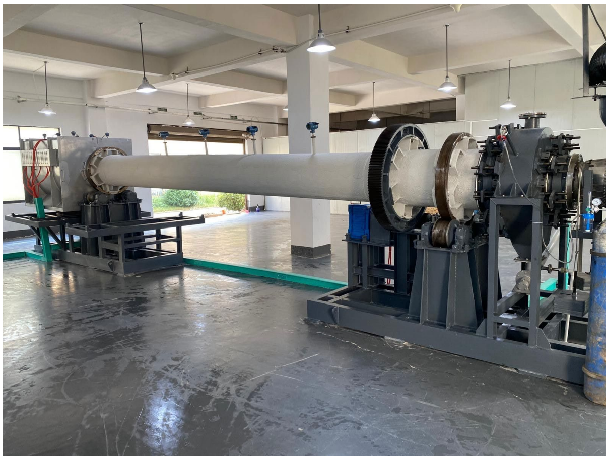
Image 1: Installation of pilot scale calcining unit at Hunan Firebird Battery Technologies' Plant
