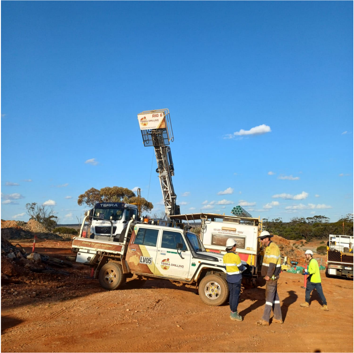
Figure 3: Diamond drill rig in operation at Mt Palmer with Terra Drilling and Kula personnel.
