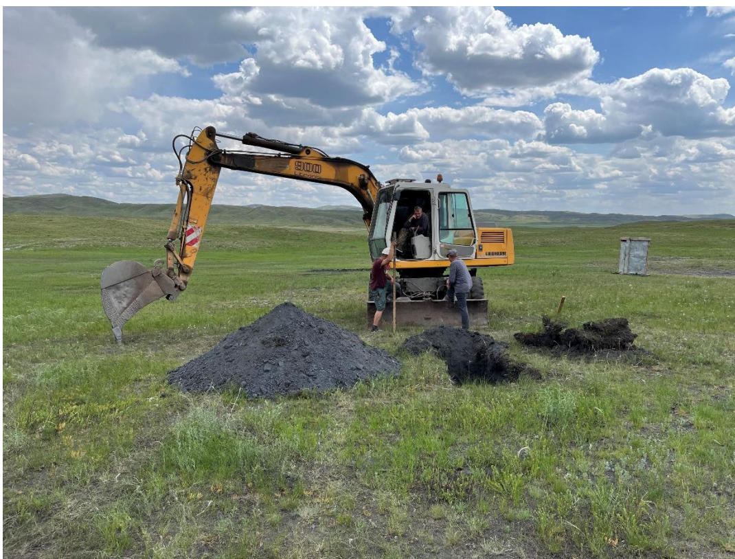
Figure 1 - Test Pitting at Sarytogan in 2022. Similar sized excavator to be used for 20t trial mine this week.
