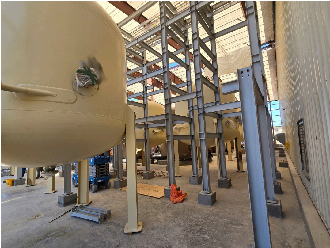
Figure 3: Ion exchange columns and pipe racks placed in new section of plant
