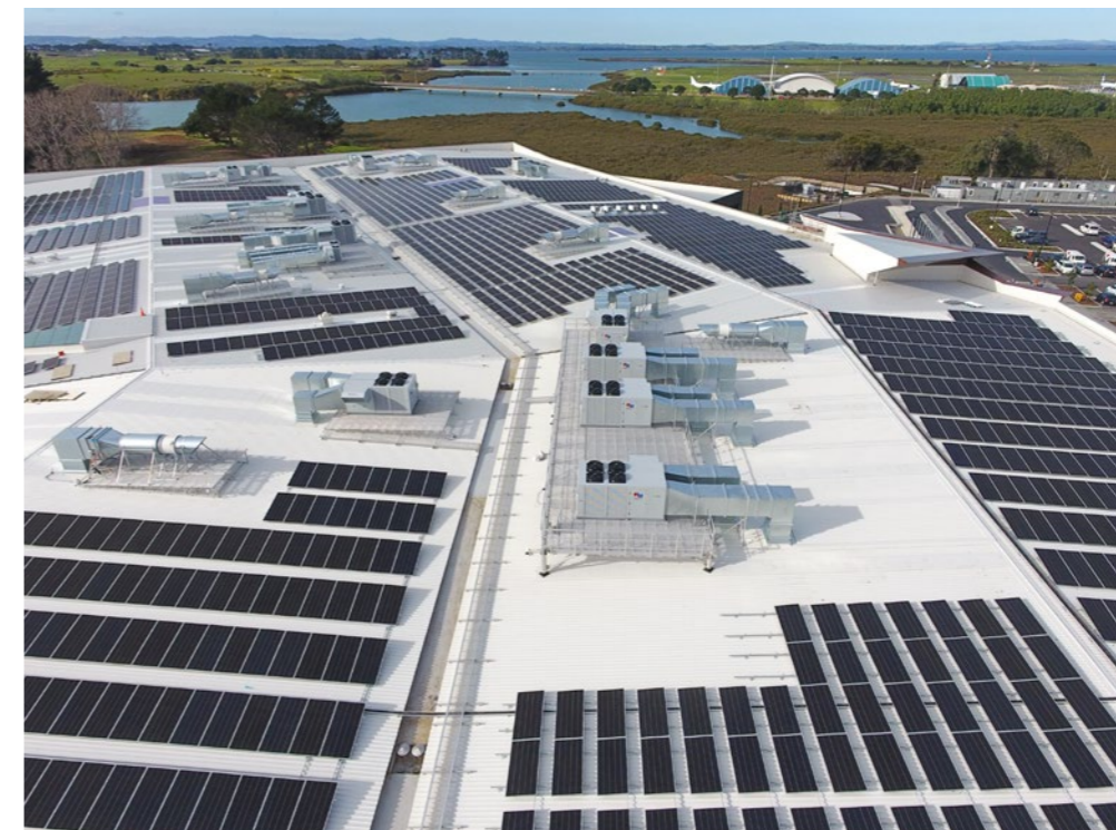
2 Rooftop solar panels on Mānawa Bay outlet shopping centre will generate 2.3 megawatts of electricity when operational in September 2024.
