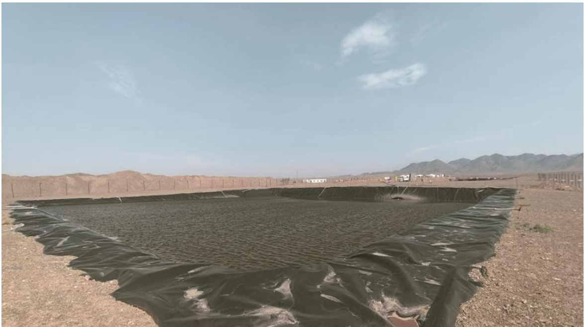
Water disposal pond at the Nomgon Pilot Plant
