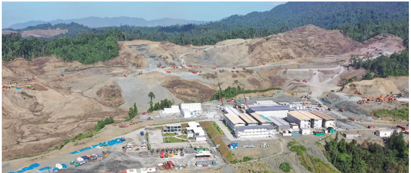
Office and staff buildings completed with earthworks and footings at ENC largely complete in readiness for concrete pouring and plant erection
