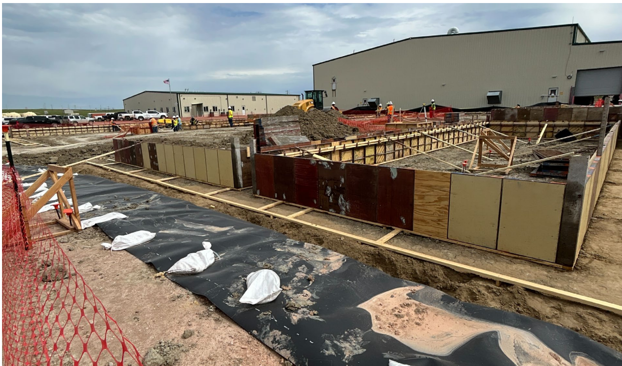
Figure 3: Crews installing forms in preparation for upcoming concrete pours at Ross CPP site
