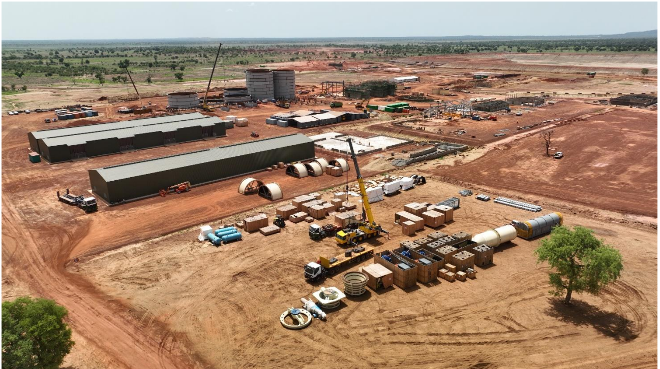
Kiaka Plant Overview (mill shells in foreground)
