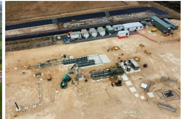
Enterprise well site
