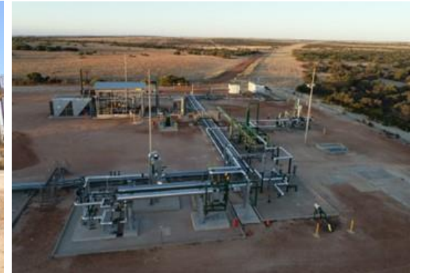
Xyris Gas Plant
