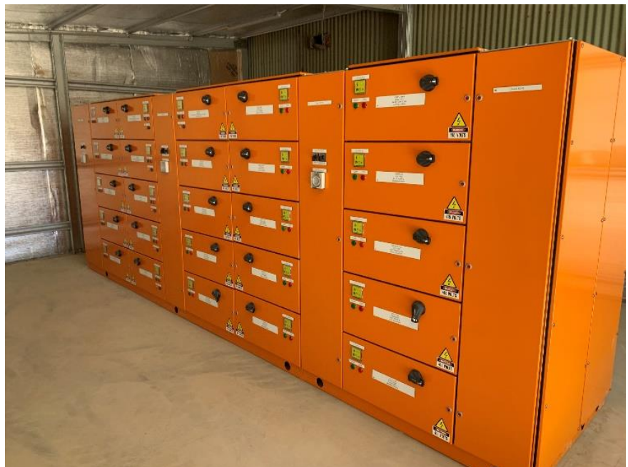
Figure 6: New motor control centre (MCC) and electrical network upgraded.
