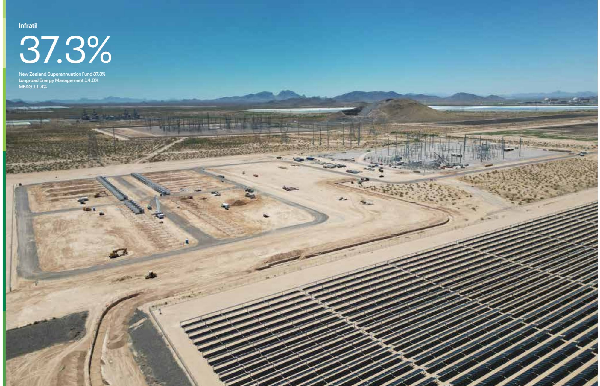
The switchyard and battery installation at the Sun Streams 4 solar farm, Arizona
