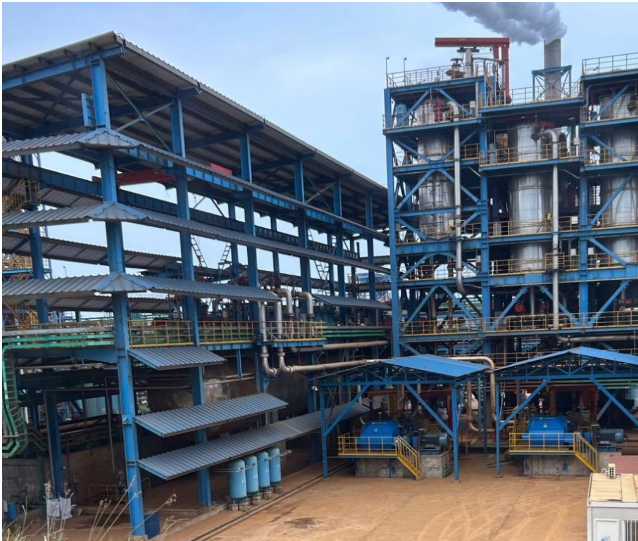
View of HNC operations
