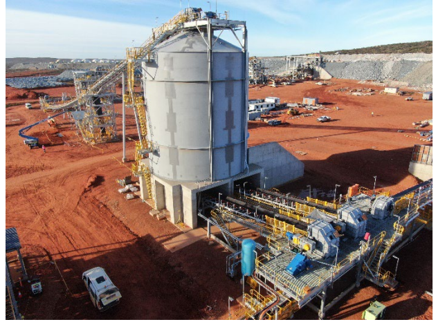
Figure 15: Fine Ore Bin and Feeders
