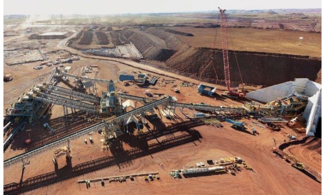
Ken's Bore crushing plant Train 3
