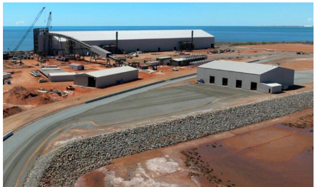
Product storage facilities at Port of Ashburton
