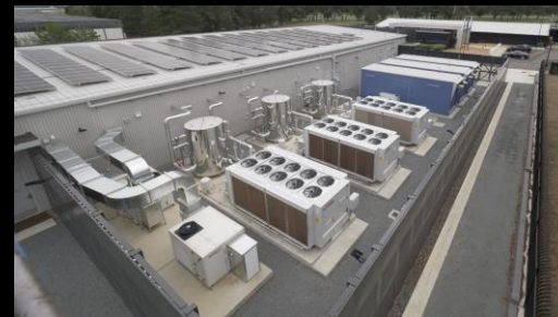
Canberra Data Centre Campus Intellicentre 4 Bunker & Intellicentre 5 Bunker
