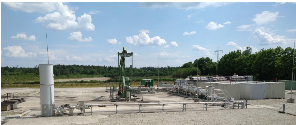
Anshof Permanent Production Facility; currently being moved from Ampfing to Anshof
