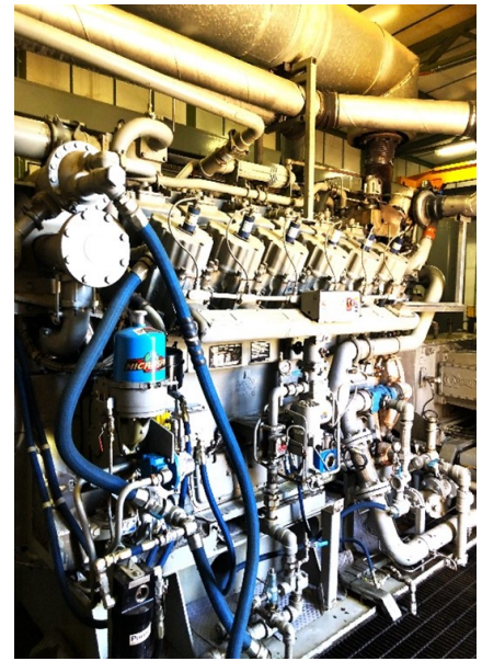
Part of the newly acquired RPGP – low pressure gas is compressed to sales gas pressure using gas engine driven reciprocating compressors
