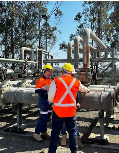
Part of the newly acquired RPGP - Gas will be delivered to the Carpentaria Gas Plant via the buried gas gathering system at low pressures to maximise well deliverability
