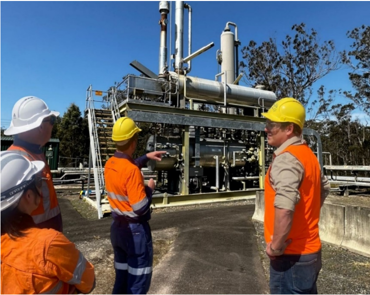
Managing Director Alex Underwood inspecting the newly acquired RPGP at the Camden Gas Project Site
