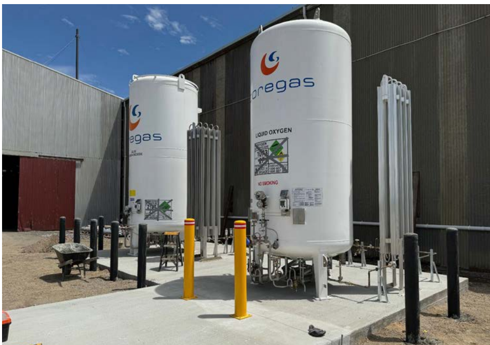
Coregas oxygen and carbon dioxide system installed
