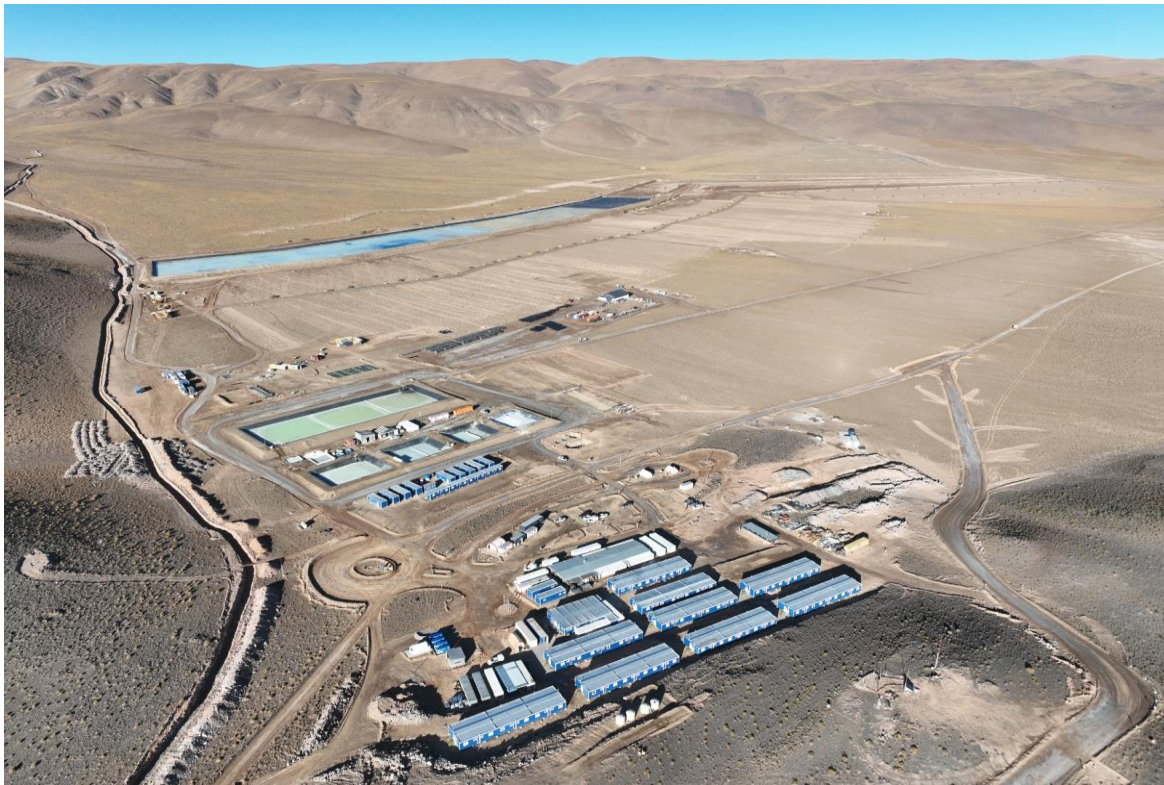
Figure 2 – Overview of HMW Phase 1 project construction (includes camp, pilot plant and filling of Pond 1 in the background)
