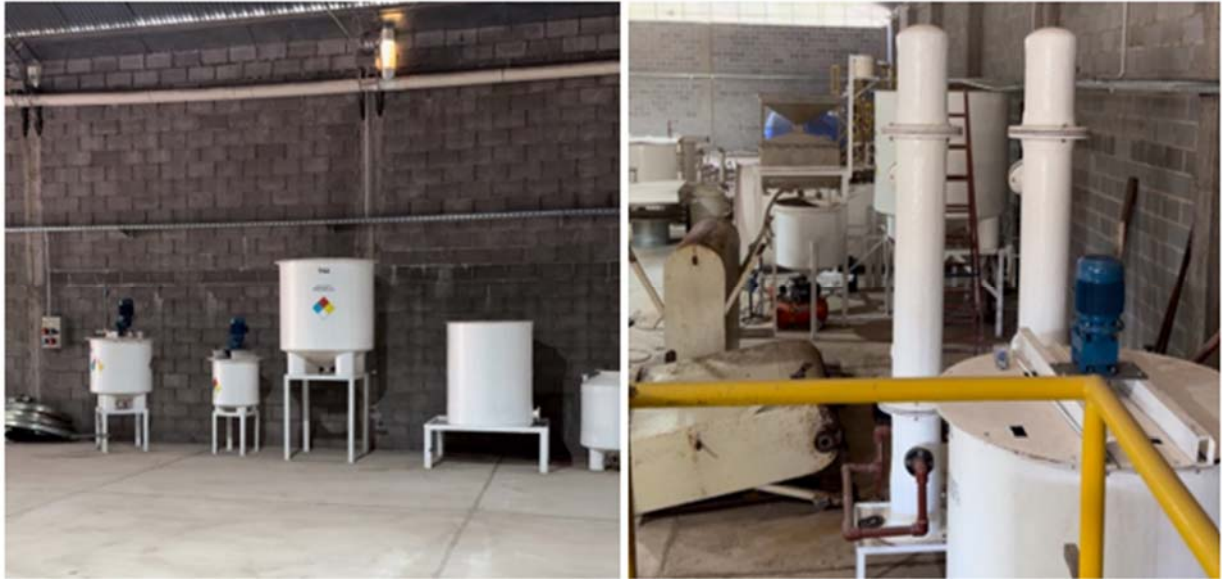
Figure 12: Plant mixing tanks and columns being refurbished at the new Pursuit Lithium Facility in Salta, Argentina
