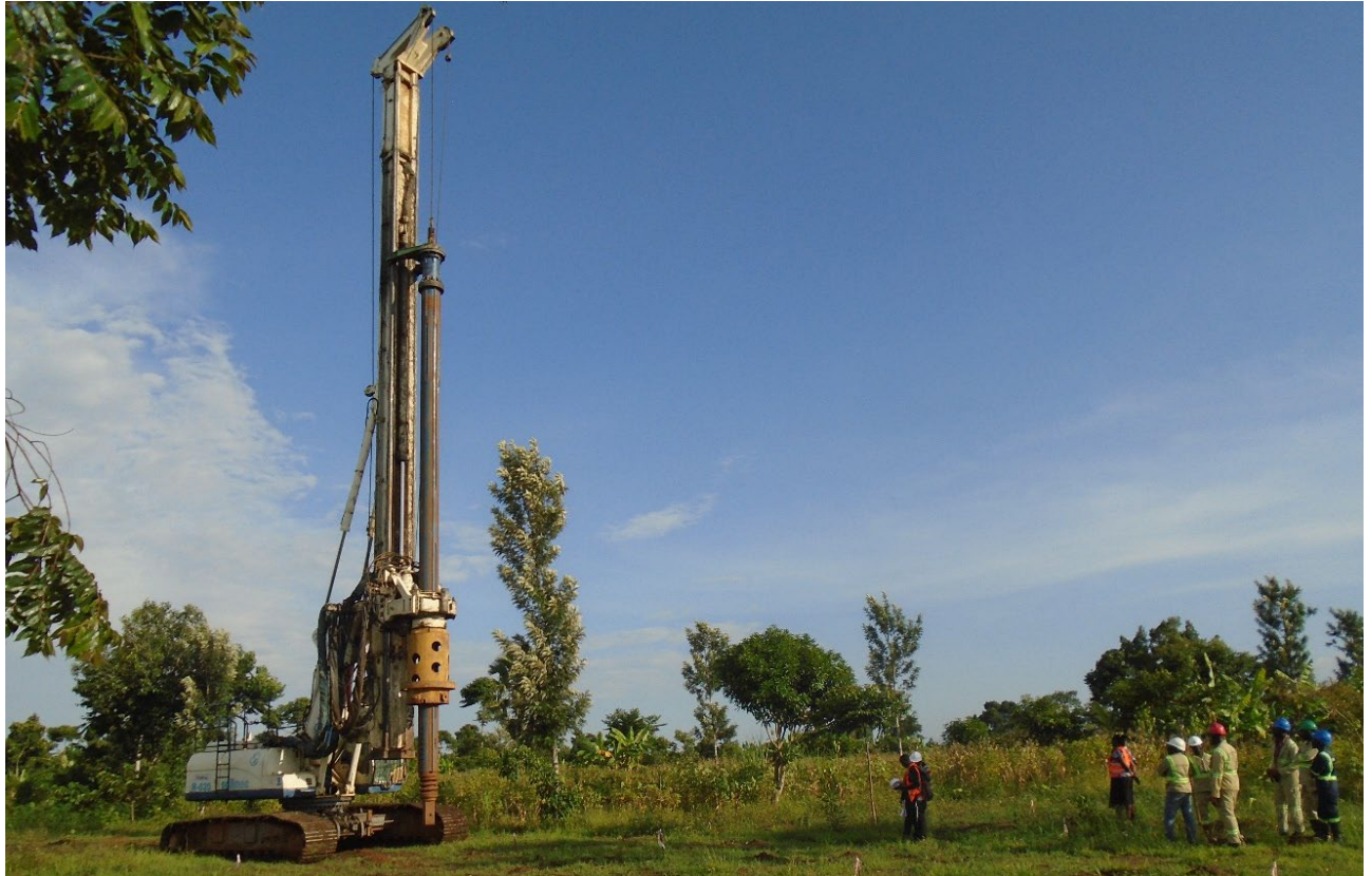
Figure 6: Auger drill mobilised to test site to collect bulk sample test material for the initial Phase 1 test program at Makuutu.
