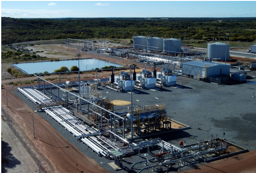
Figure 6: ASP processing facilities
