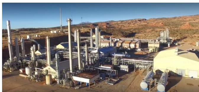
Figure 2: “5.5 Nines” Lisbon Valley Gas Processing Plant.
