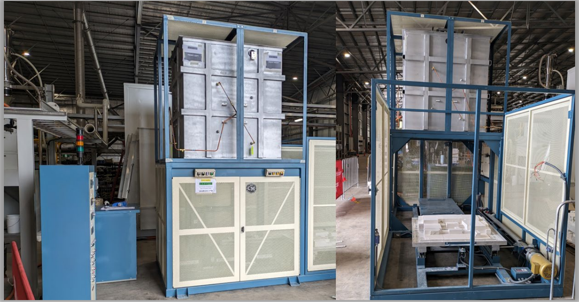
Sinter oven for HPA tablets – installed and in commissioning
