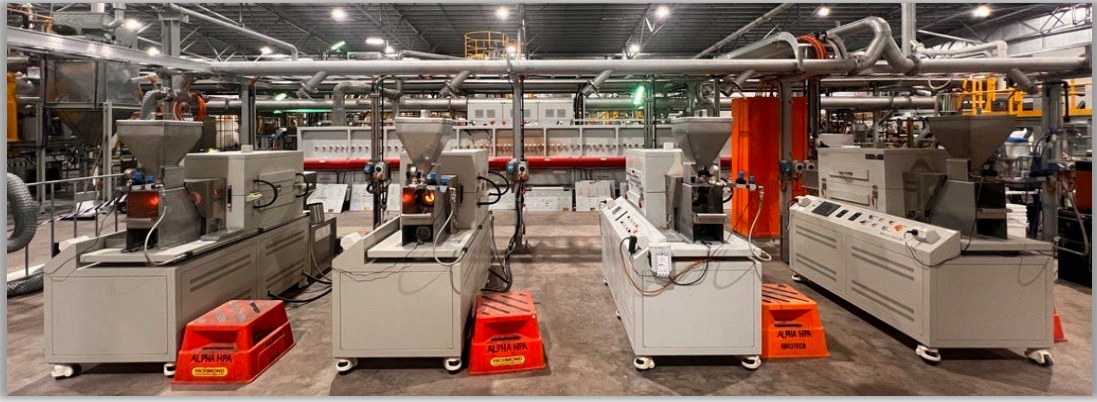
HPA rotary kilns – in final commissioning
