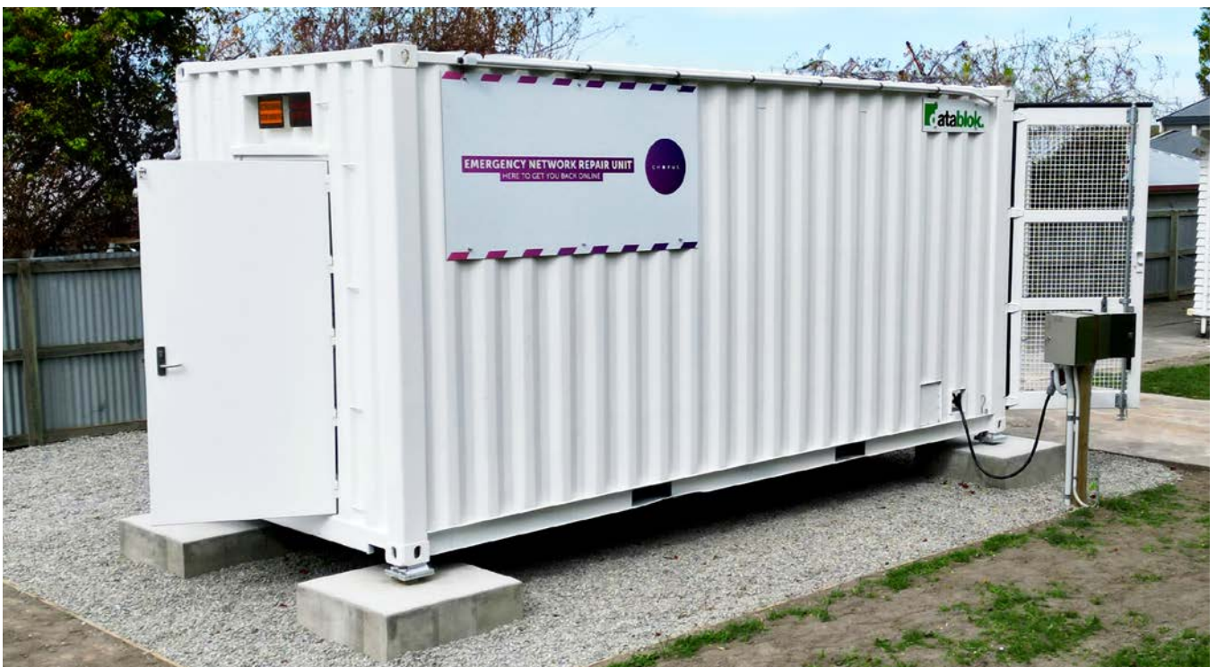
Two containerised emergency exchanges have been built and are on standby for future disasters. One is stored in the North Island and the other in the South Island.
