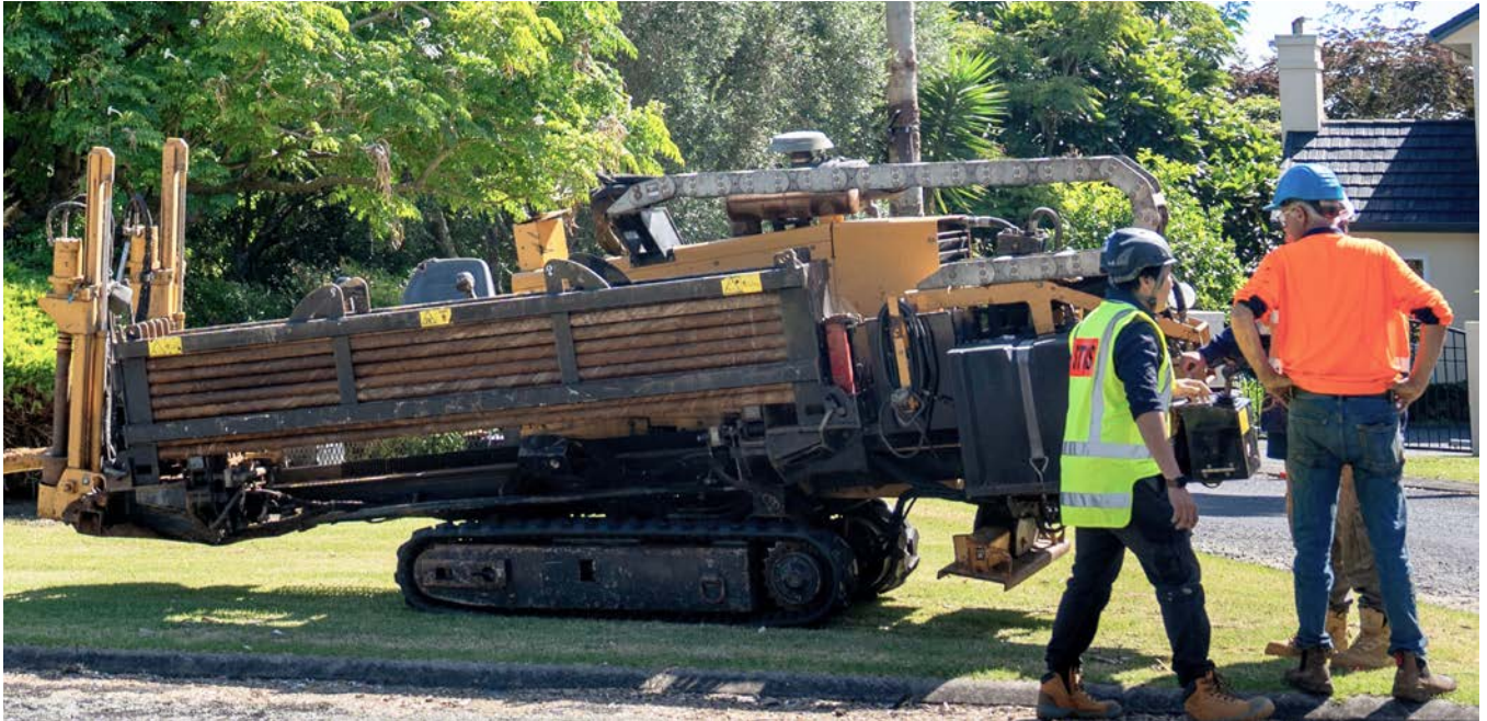
An underground directional drilling machine in Waiau Pa, South Auckland, for the recently announced fibre rollout.
