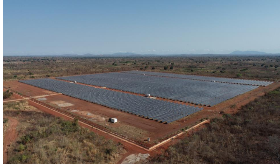
11.25 MWp solar photovoltaic array
