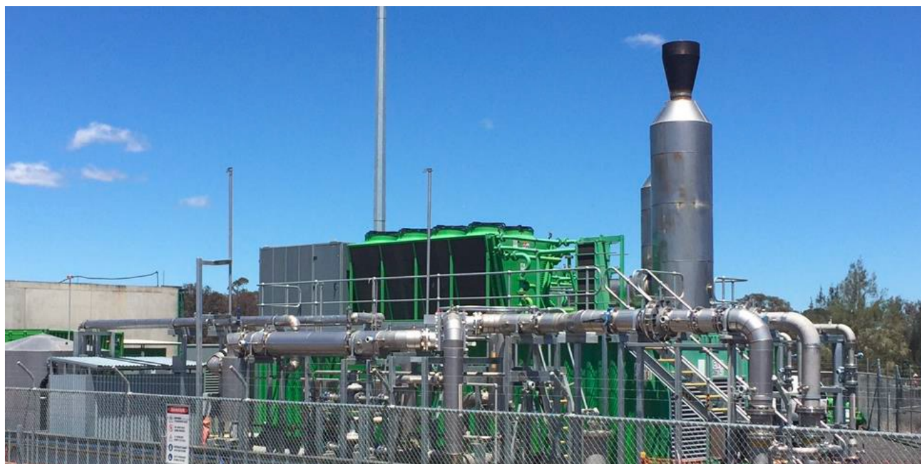
Landfill Gas to Power Generation Facility, Western Sydney – TSF Power
