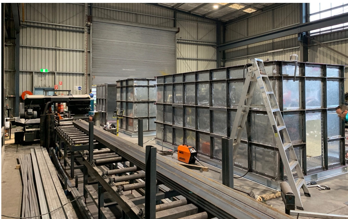
Damper Balance Tanks – Tank Industries
