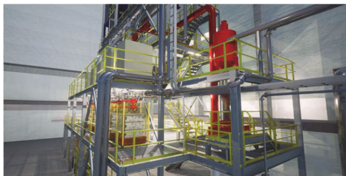
Figure 6: In-house designed packed bed calciners
