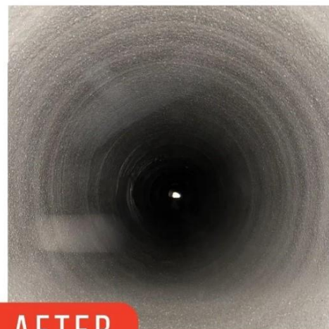
Figure 3. Worn pipeline after re-habilitation
