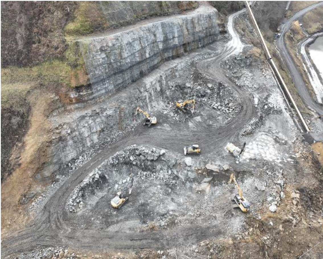
Image: Excavation works on the new surface raw coal stockpile at Buchanan
