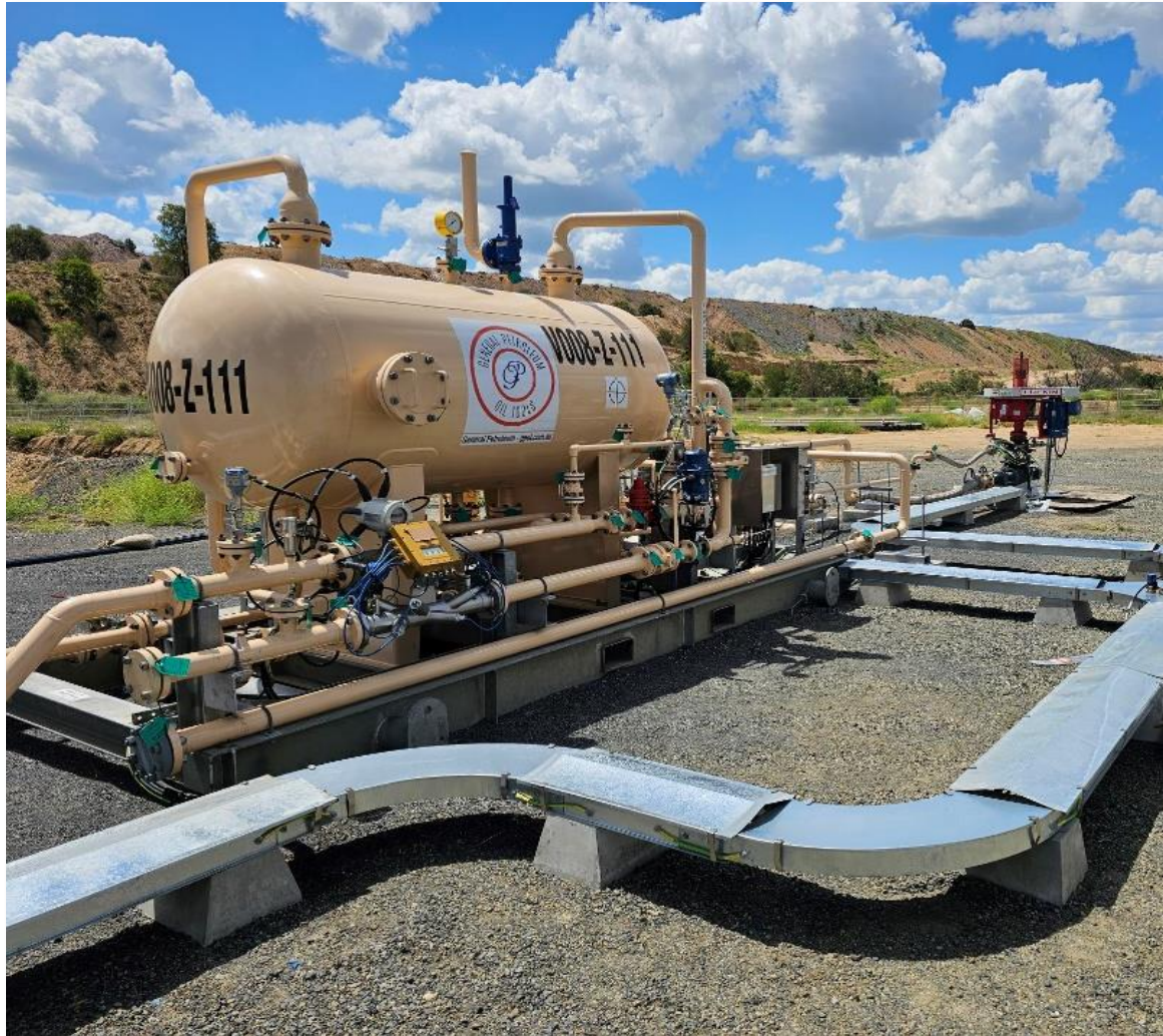
Image: Curragh Gas Project surface infrastructure
