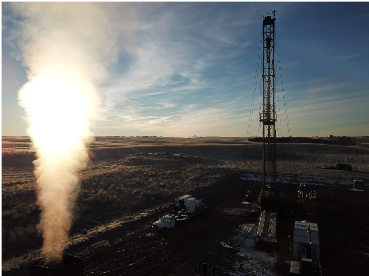
Figure 1: Jesse-1A flare-stack venting reservoir gas and helium to surface during flow-testing
