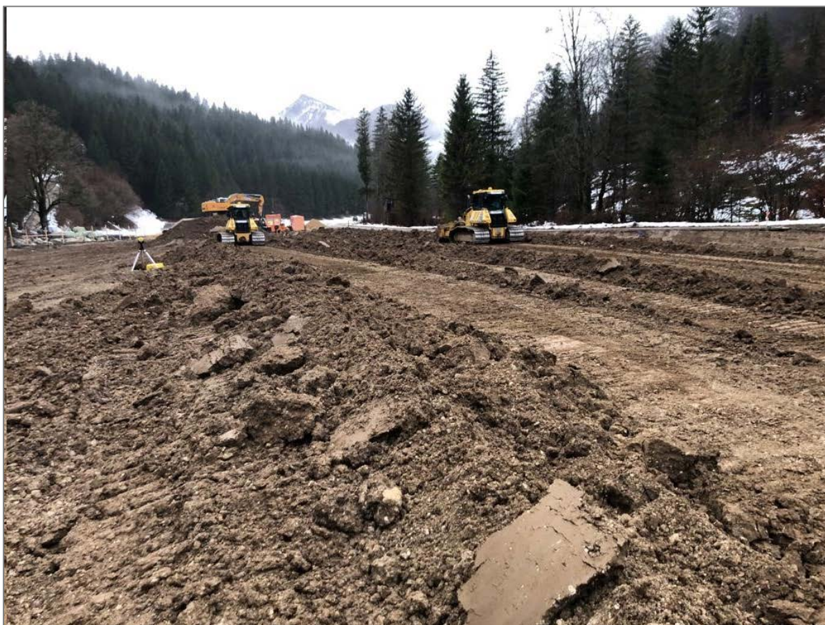
Well construction operations clearing top soil before installation of foundation material for drilling at the Welchau-1 well site
