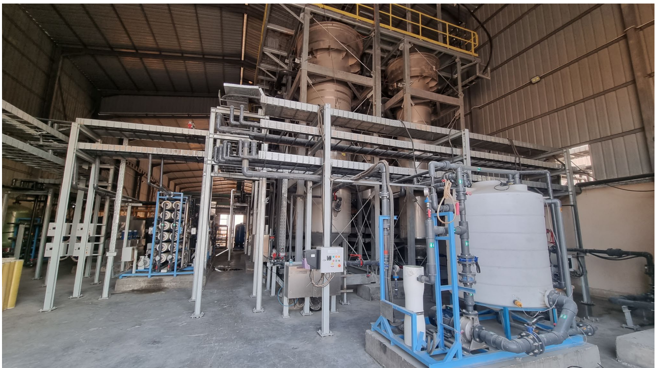
Picture of the completed HIROX ® Plant in the Middle East
