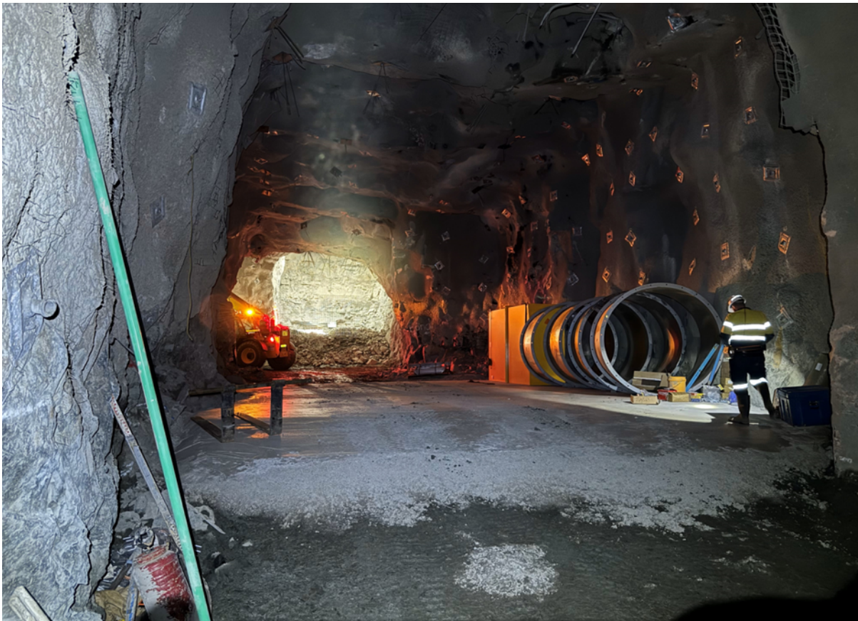
Figure 6 - Underground at Riverina showing the 4.5m diameter vent rise in the background and the cement pad poured as part of the primary fan installation (scheduled completion early December)
