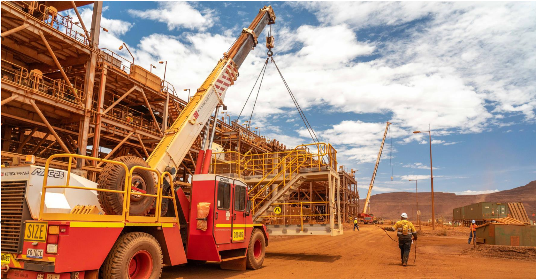
Monadelphous undertaking maintenance services at Fortescue's Solomon mine, Pilbara region, Western Australia.
