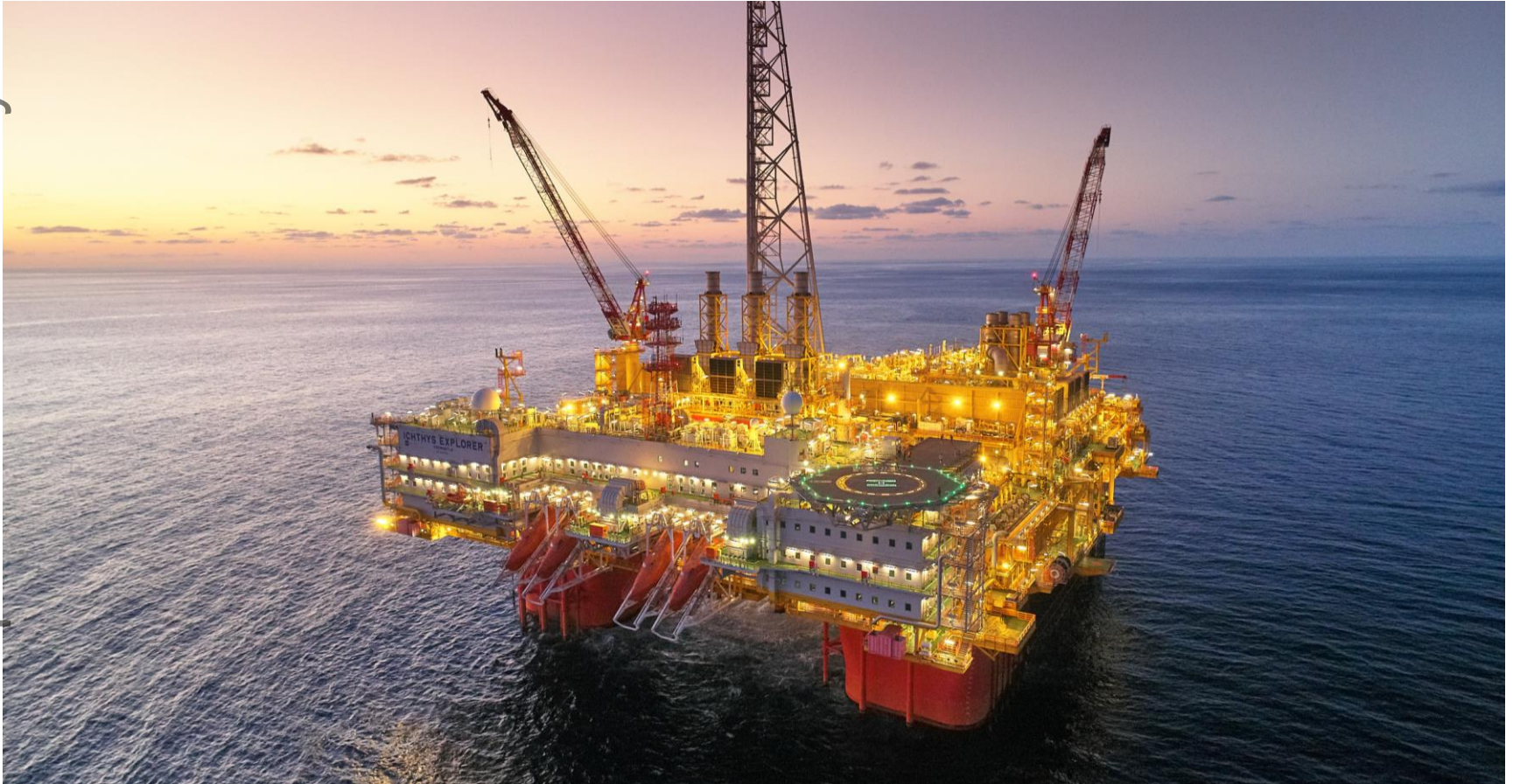
INPEX's Ichthys Explorer central processing facility, located in the Browse Basin, approximately 450 kilometres from Broome, Western Australia.
